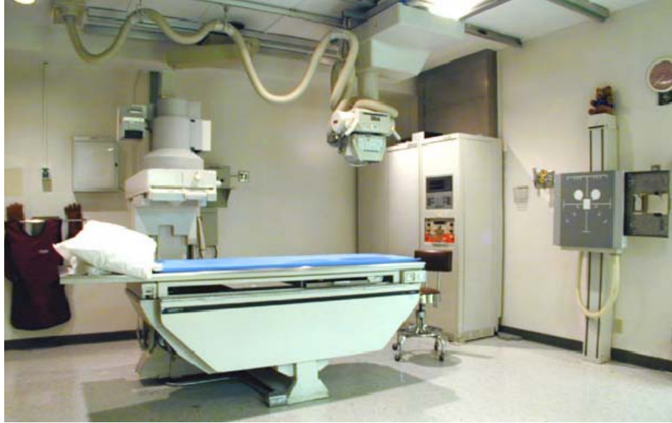
Figure 2-2. Another view of the working side of the X-ray table.
